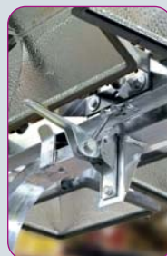
Anchoring for lamps
