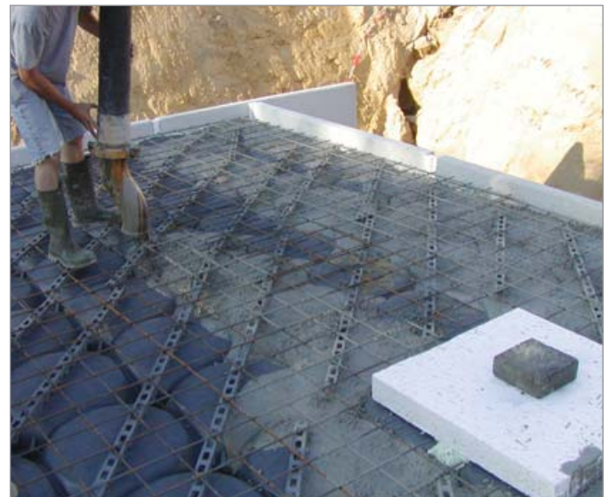
Dispersion tank under a residential area
