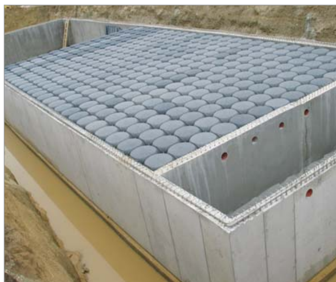
Water collection tank under an industrial area
