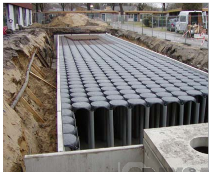
Dispersion tank under a residential area
