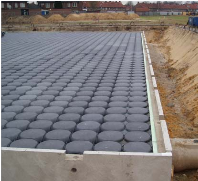
Collection tank under a green area
