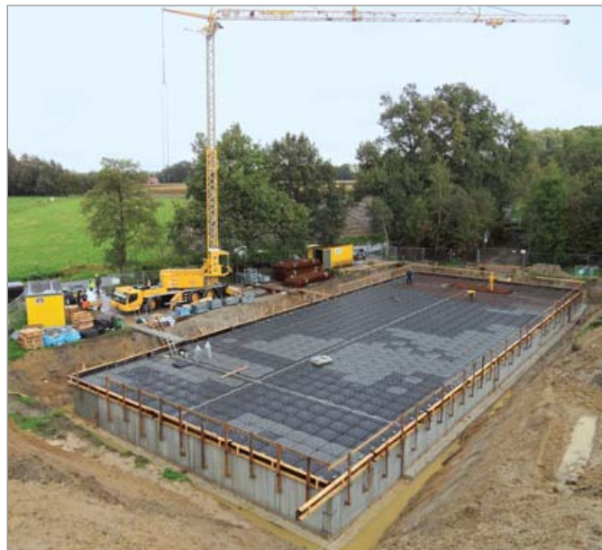
Water collection tank
