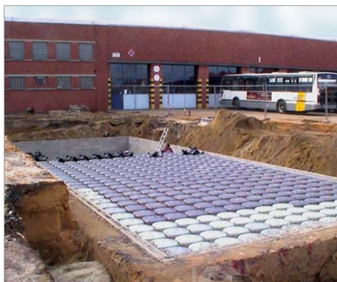
Collection tank under a parking lot
