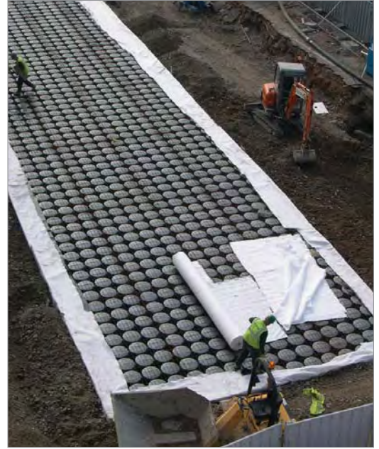
Water collection tank
