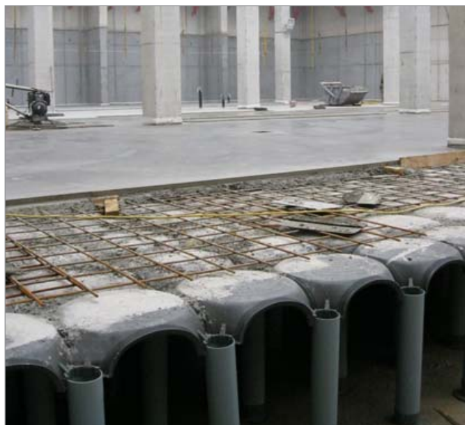
Eni Green Data Center
