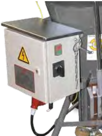
In the central control cabinet, the electrical system is easily accessible at all times – which makes maintenance work easier.
