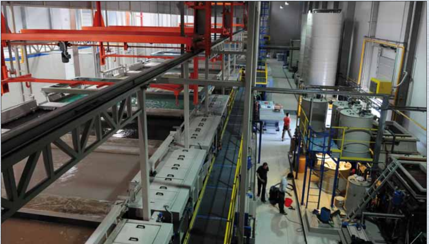
environmentally friendly cataphoretic painting system in production plant SK-Cont, SK-Komarno
